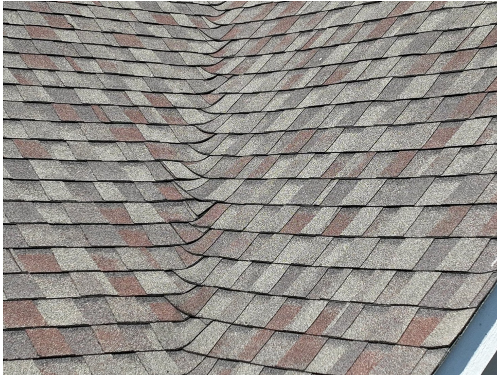
Fig. 5 — Shingle field, close frame: granule coverage uniform; the pronounced shadow lines along tab edges are the condition noted in the findings table.
